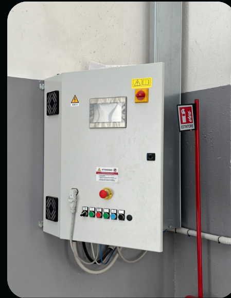
panel de control 4.0
