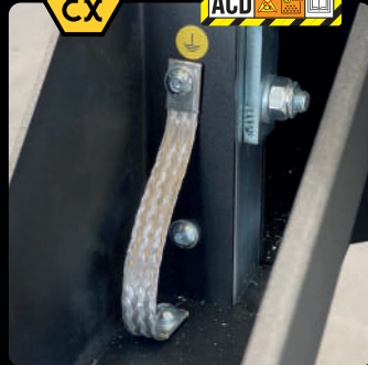
ALL COMPONENTS ARE GROUNDED
